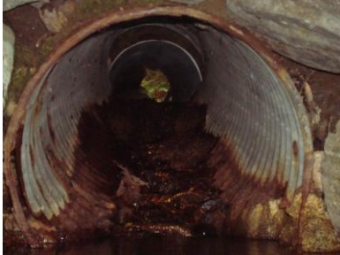
Culvert showing corrosion from stormwater
